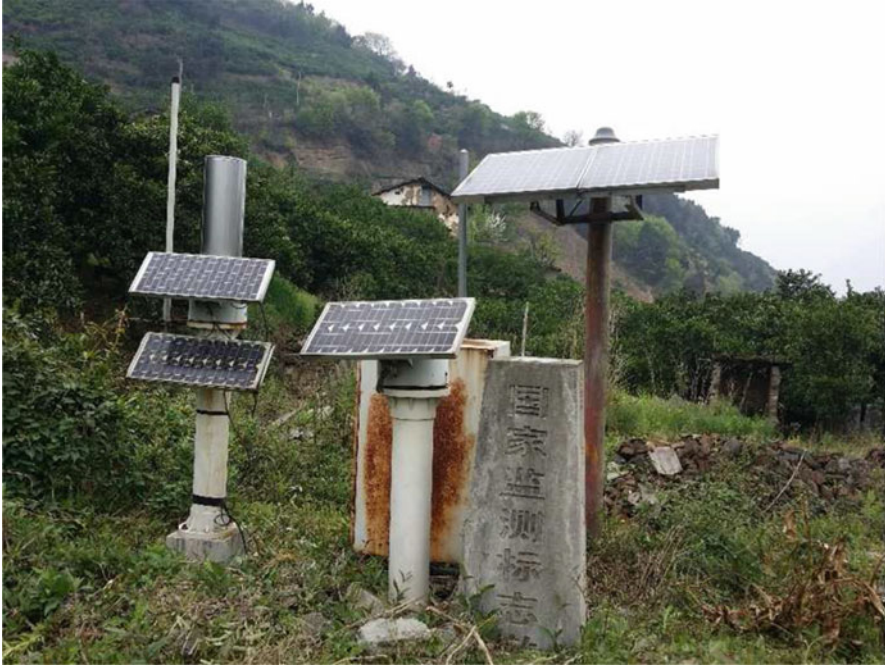
Fig. 3.5 Detecting rain gauge and deep deformation
