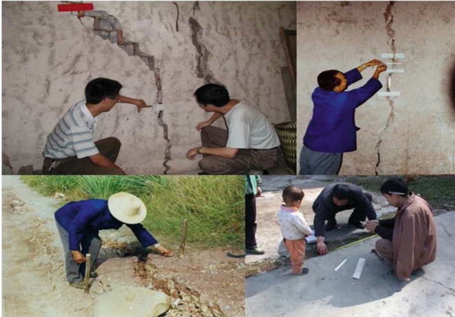
Fig. 3.9 Scraps of paper to monitor wall crack (the upper figures) and a tape to measure the length of landslide rupture (the lower figures)
